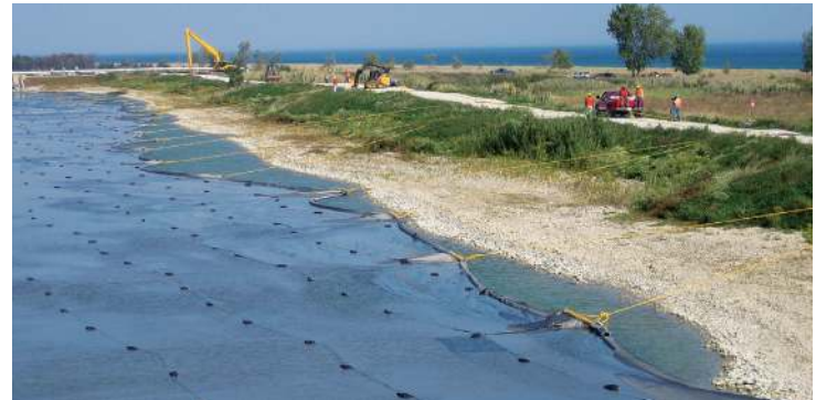
High seam strengths are critical to the field performance of the panels to prevent rupture during fill placement over the low-bearing capacity sludge/ash.
